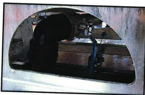
Picture 20: Tank total drain shut-off valve.
