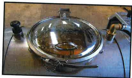
Picture 21: Tank filling valve
